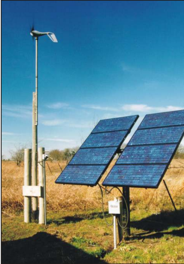
An Air 403 pairs with a PV system to supply a consistent supply of power for battery charging.
